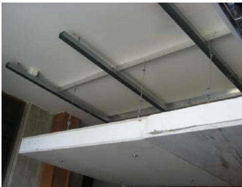
Fig. 2. H/C radiative ceiling panels with panel assembly
