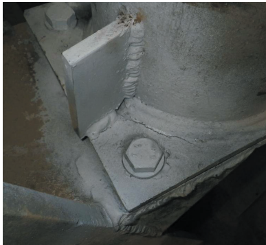
Fig. 3. Fatigue crack in the side bracing
