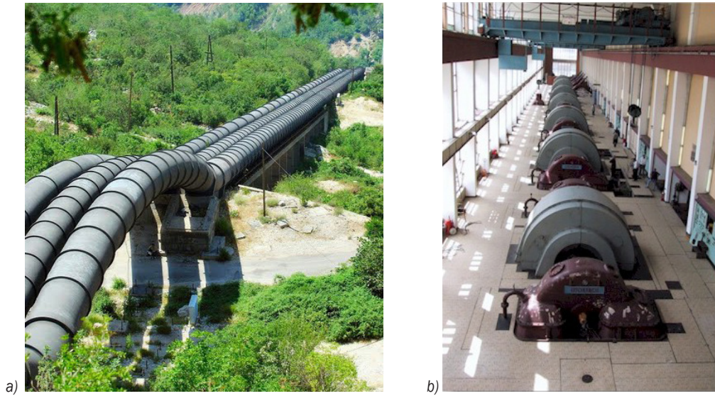
Fig. 3. Layout of a) three parallel penstocks and b) powerhouse with seven twin-type Pelton units in Perućica HPP
